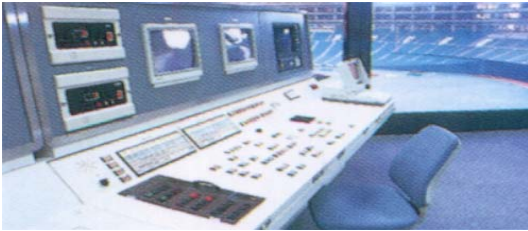
Systems for public buildings
